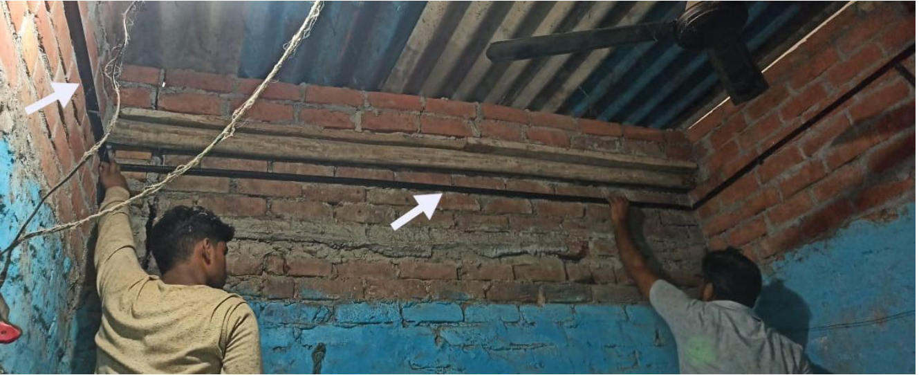
Figure 2.16: MS L-angle drilled at a height of 14" approx(in this instance) from top of wall on all 4 walls to form the support frame
