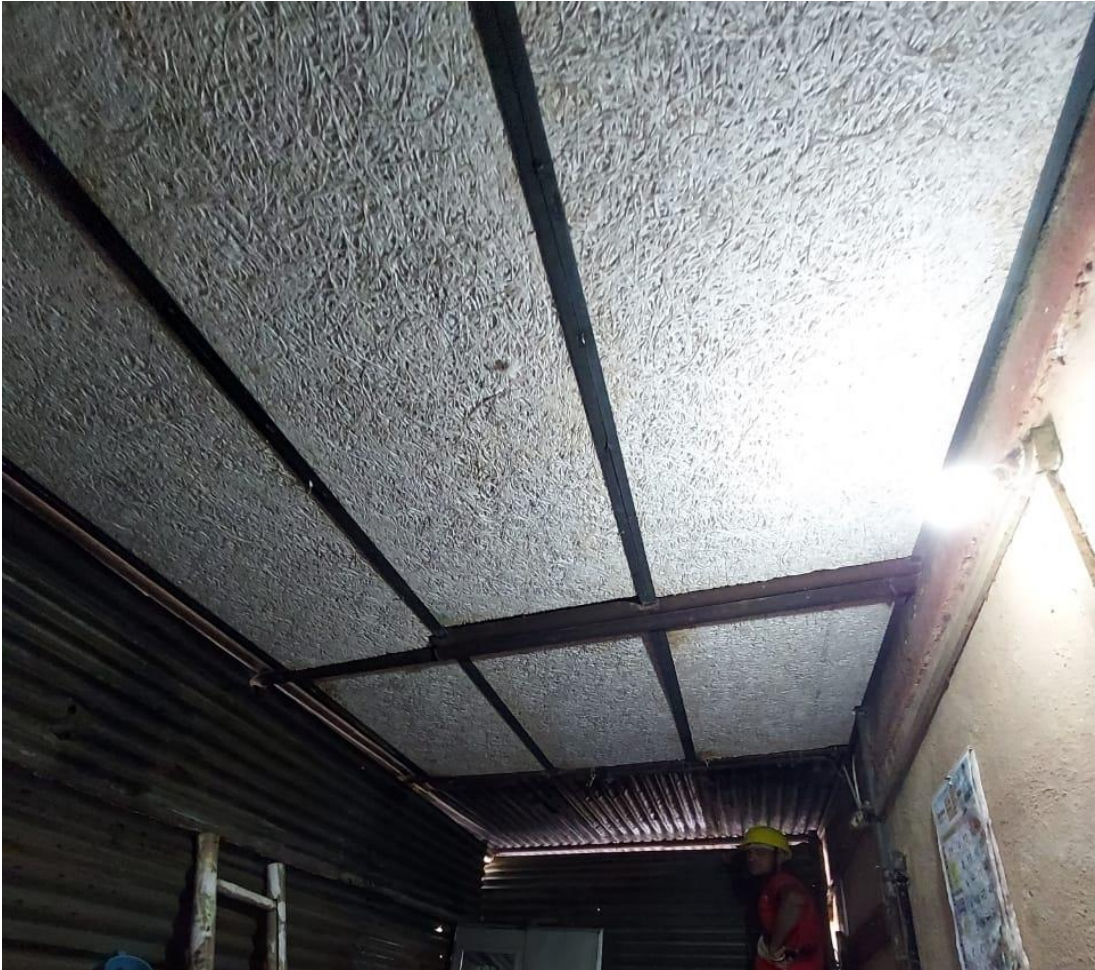
Figure 3.5: MS support framework with panels in place
