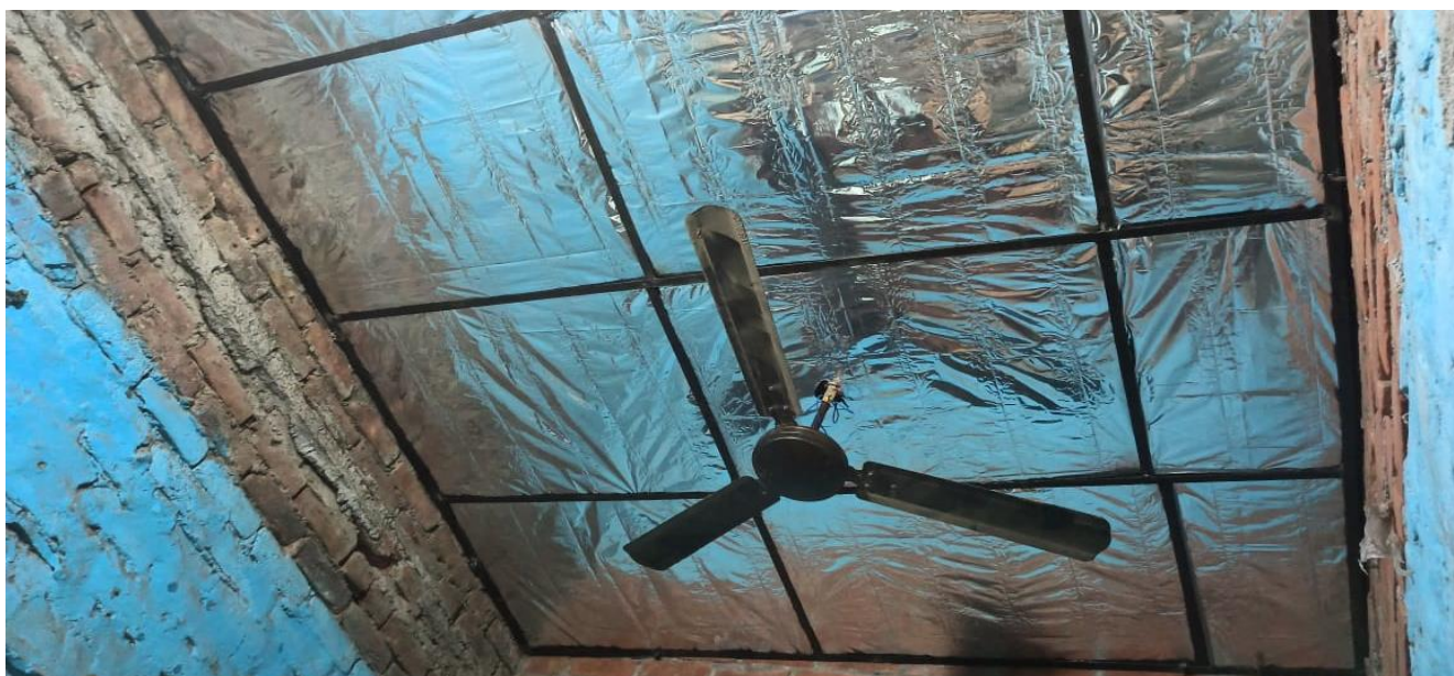
Figure 2.21 Metal support framework with panels in place with no gap in the ends
