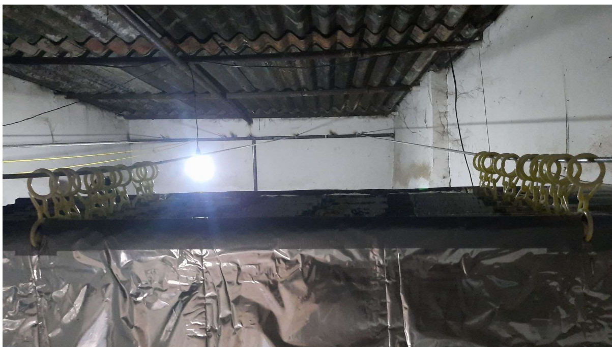
Fig 37.1.3-2 : Top View post hooking the IDB fractal on the steel wire.
