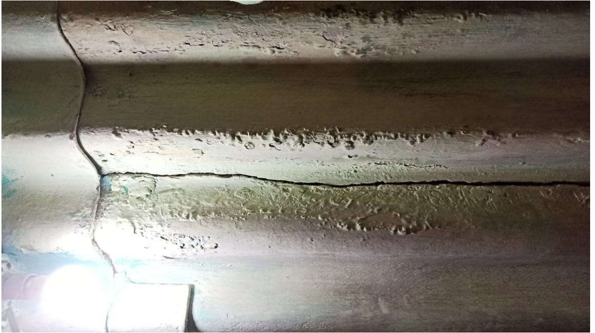
Fig 25.2.1.7-1 : Crack in the Roof
