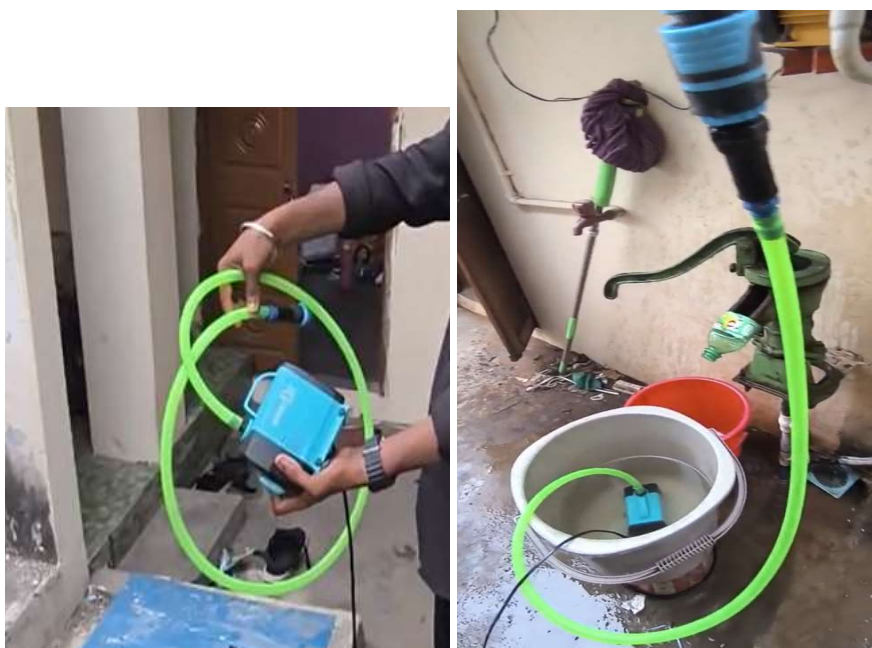
Fig 35.3.2-4 : Submersible Pump Connected with Hosepipe
