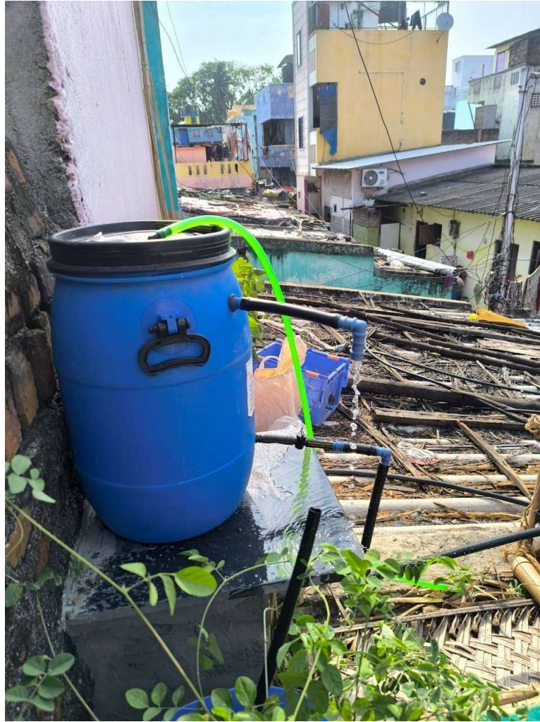
Fig 37.4.2-18 : Water over flowing through the Tank's outlet
